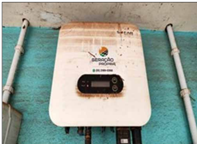
Figure 2. Inverter damaged by flooding.
